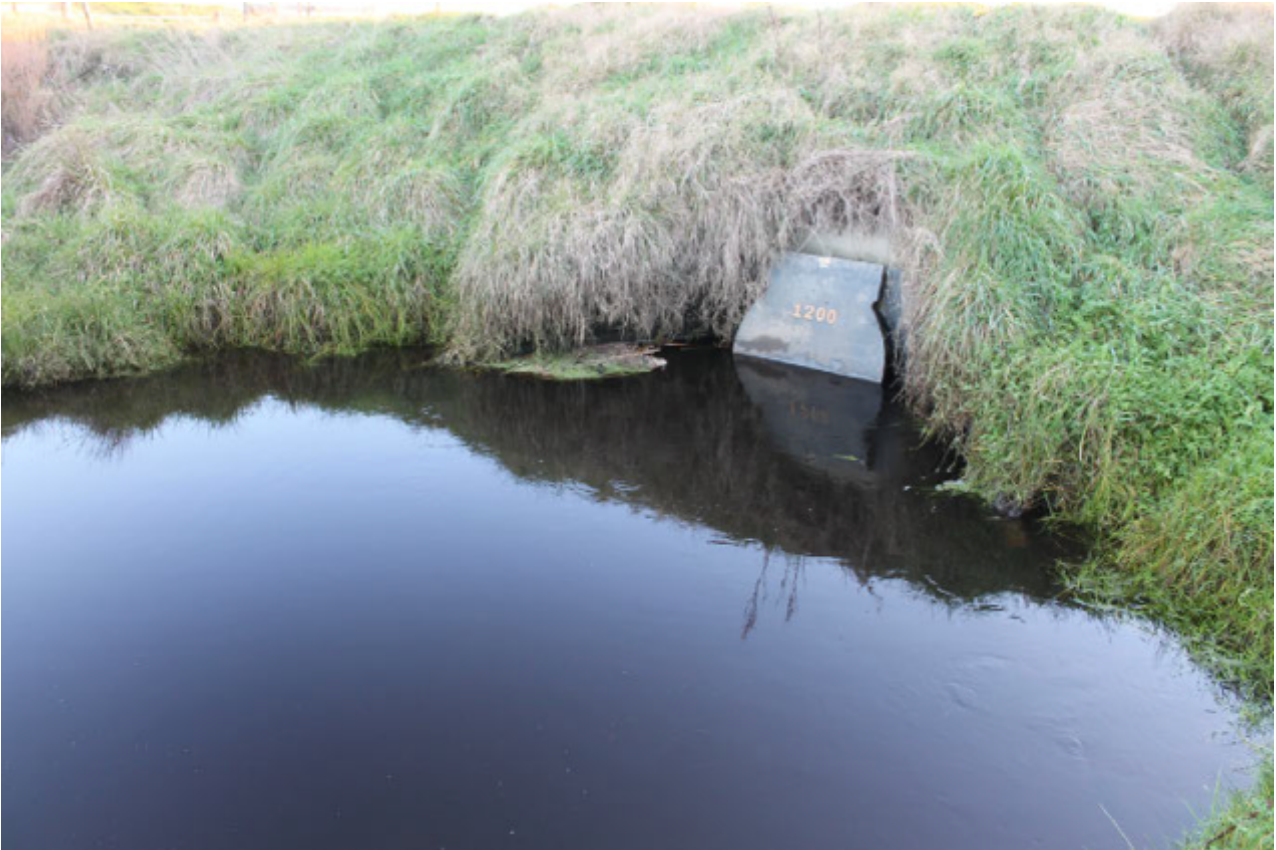
Figure A.17: Flood Gate exiting via culvert, under stop bank and into the Ōhau River from the Loop terminus. Image Hayden Fowler 2021.
