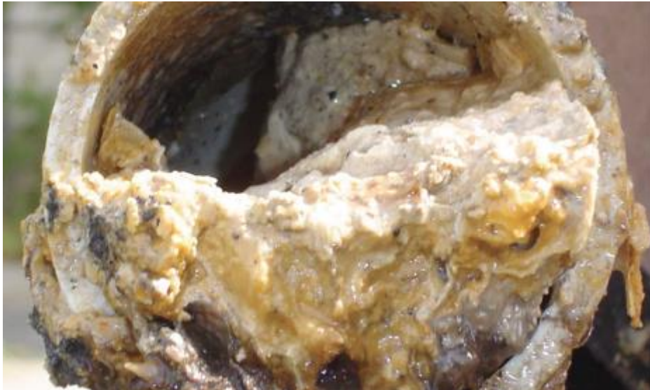
Figure 4.8: Fat, oil and grease build up in wastewater pipeline, Severn Trent, UK (Source: Guardian 12 Dec 2016)
