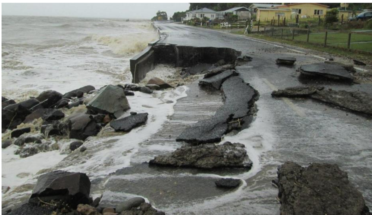
Figure 4.4: Damage to road at Whakatete Bay due to coastal flooding and wave overtopping (Source: Meghann Rawlings)
