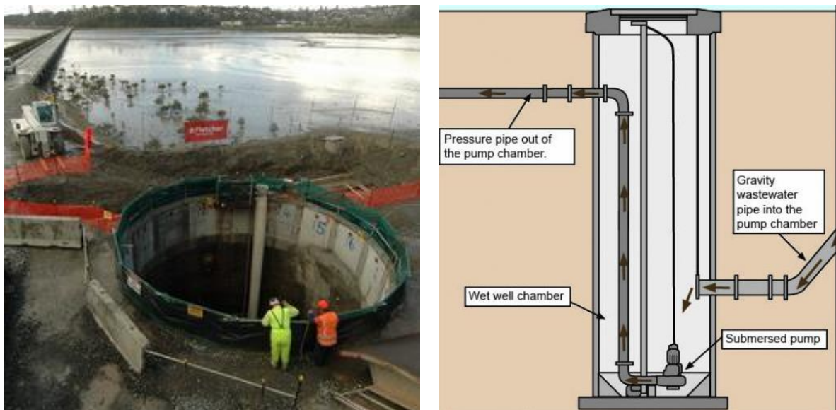
Figure 3.12: Project Hobson pump station, left (Fletcher Construction, 2010), and example pump station, right (Rebuild Christchurch, 2015)
